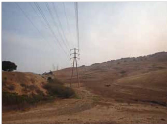
PHOTO 3: Western Power Line.
