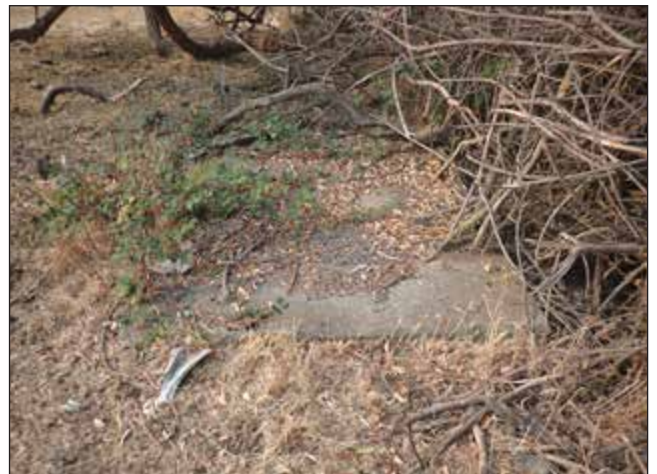
PHOTO 4: Water Main Covers
