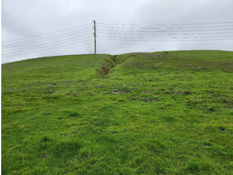
View looking west of a graded commercial pad with an erosion gully in a pasture setting
