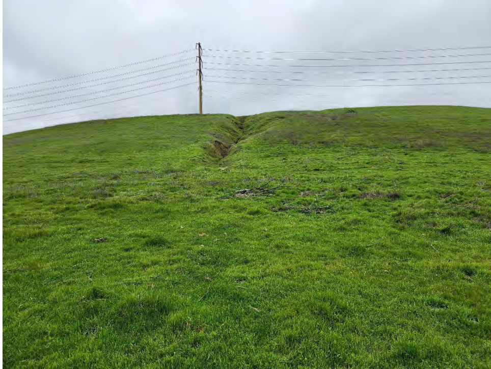
View looking west of a graded commercial pad with an erosion gully in a pasture setting
